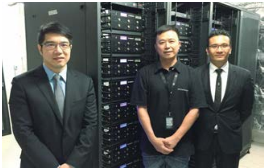
Sala de equipos y grabadores de videovigilancia. Kevin Iek (Director of Surveillance Technology), Raymond Ho (Sales Engineer, Dallmeier International), Roberto Leong (Manager of Surveillance Systems)
